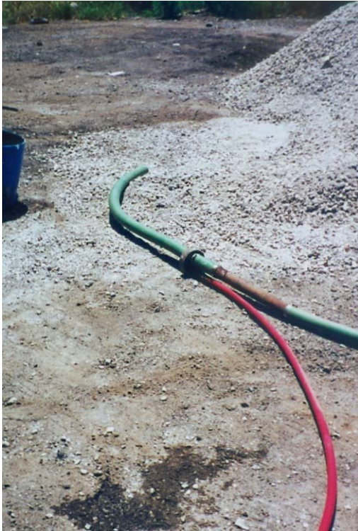
JET HOSE ATTACHED TO JET PUMP
